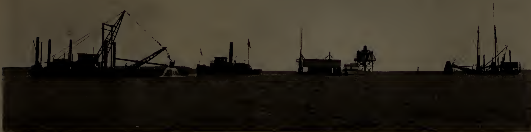
PLANT OF THE EASTERN DREDGING COMPANY, Contractors for River, Harbor, and Dock Improvements.
